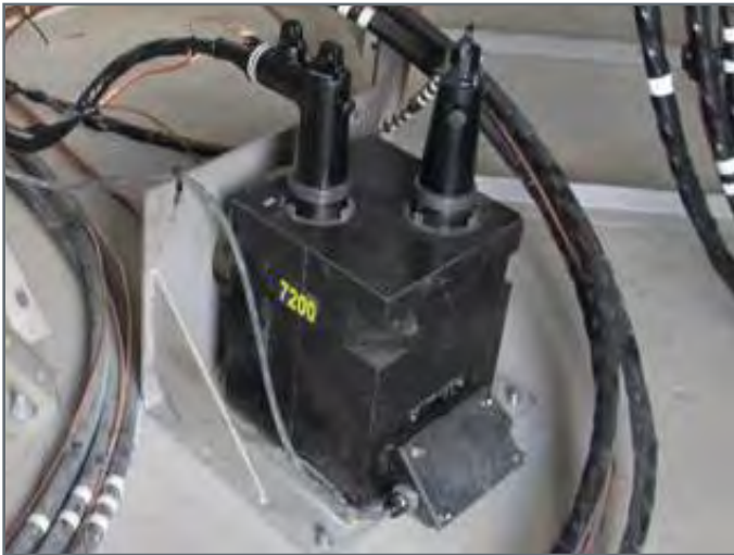
▲ Example of integrated external transformer
