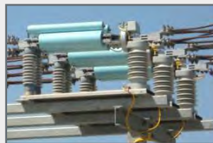
System Protection Equipment
